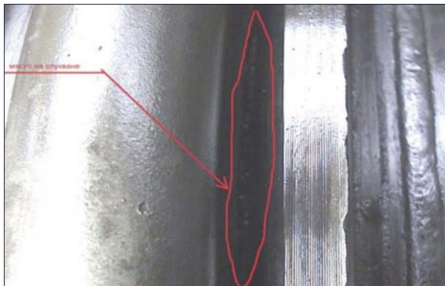
The red circle indicates the heat exchanger compensator crack (Fig. 10).
