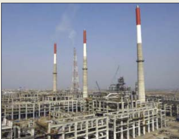
The new sulfur-processing unit mirrors the original unit, built in 1999, except that it recovers more sulfur, conforming to newer environmental regulations. Photo from Black & Veatch.
